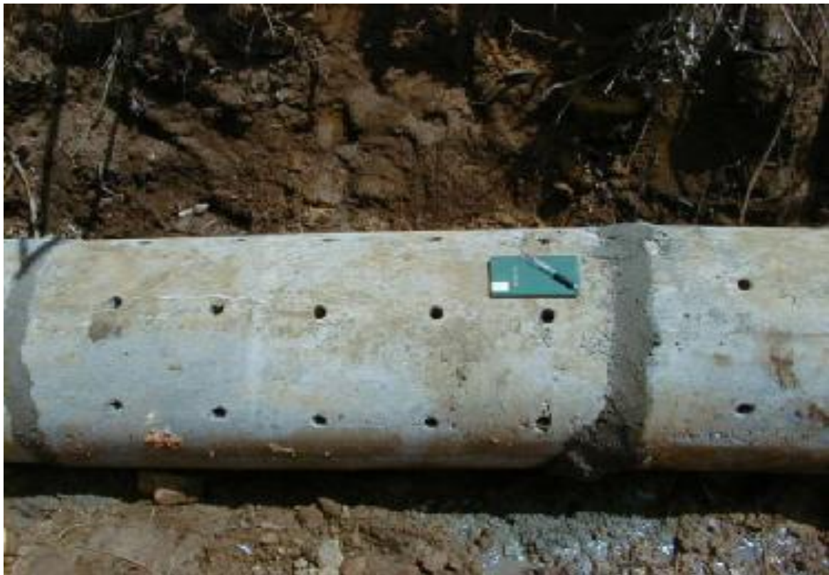
Fig. 7 Wastewater collection Pipes net works
