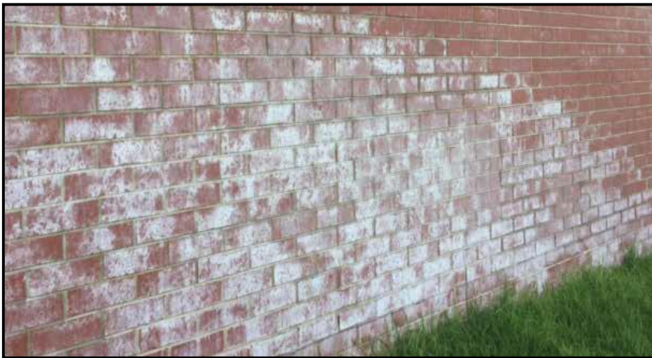
Efflorescence on brickwork
