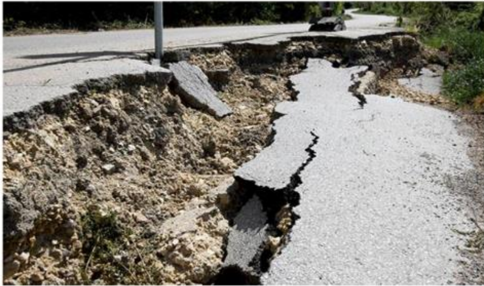
Figure shows a road constructed on a collapsible soil.
