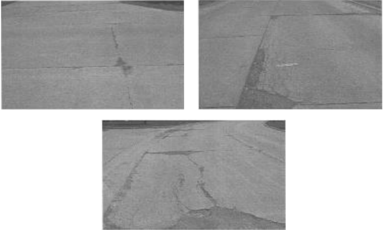
Figure (13-C) Durability Cracking.
