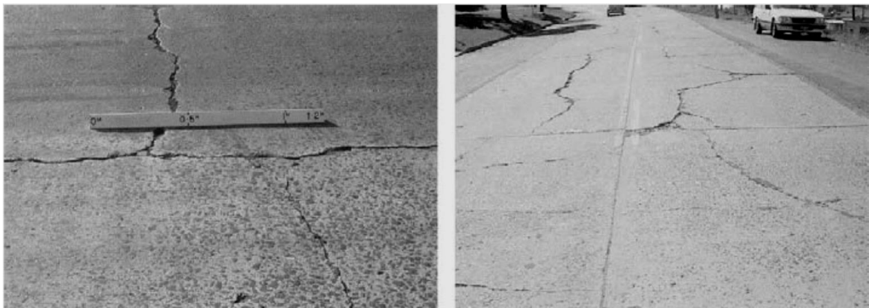
Figure (7-C) Block cracks in rigid pavement
