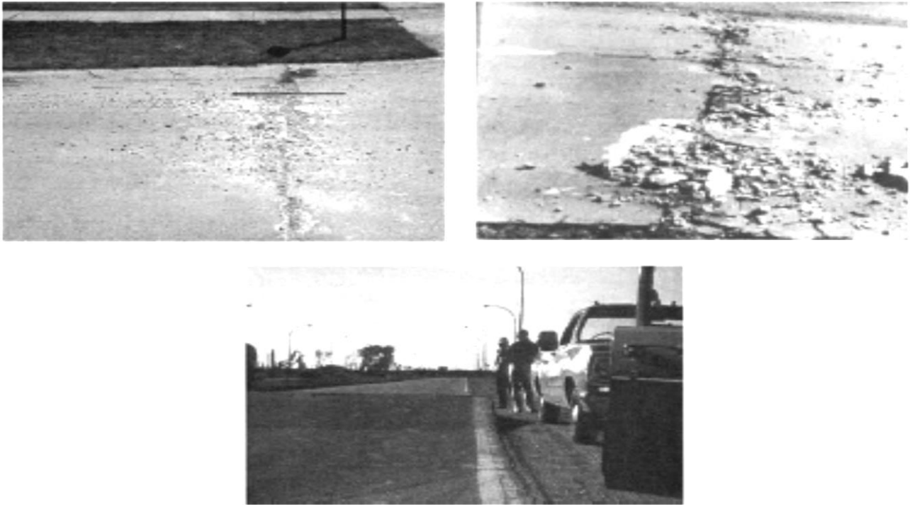
Figure (5-C) Blowup/Buckling
