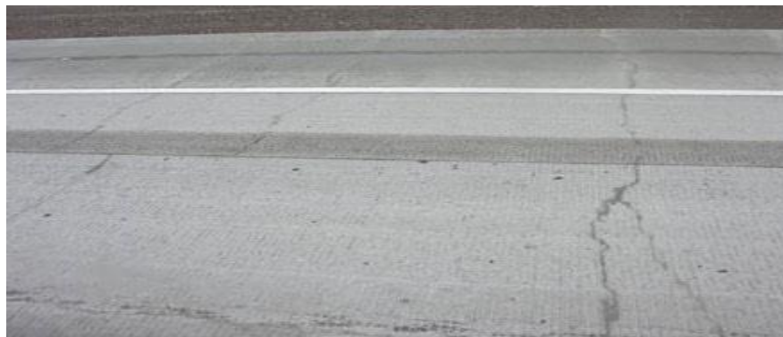
Fig.9: Cracking of Continuous Reinforced Concrete Pavement
