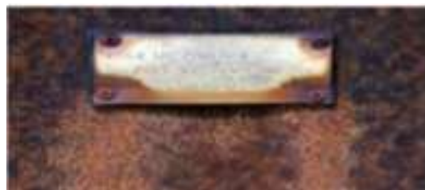
Galvanic corrosion between Steel and Brass.
