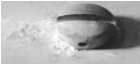
Galvanic corrosion between stainless steel screw and Aluminium
